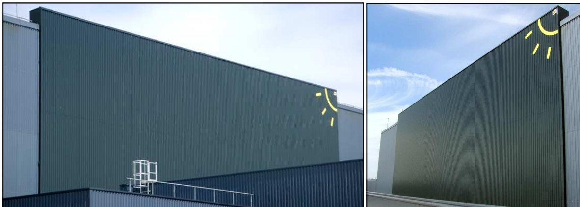
Two different views of the SolarWall® system at TMMF's plant in Valenciennes, France
